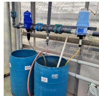
Double check injection ratio and stock tank mixing rates. Calibrate injectors and test diluted EC.
